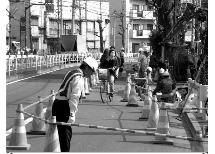
Gradbišče v Tokiu. Policista so prav posebej namestili, da bi se zaradi neprijetnega obvoza opravičeval vsakemu mimoidočemu posebej. Construction site in Tokyo. A police officer was stationed for the sole purpose of personally apologizing to each passer-by for the inconvenience of the detour.
